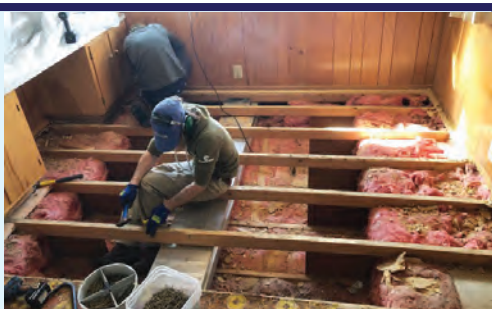
Conor and Xander from COVER replacing the subfloor in a mobile home severely damaged by a hot water heater leak.
